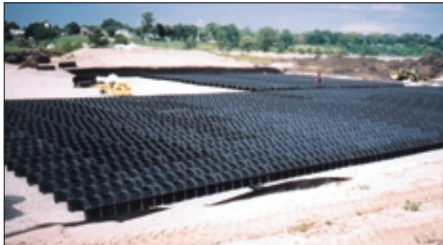
The exfiltration gallery at the Port Burwell Sewage Treatment Plant in Bayham, Ontario includes approximately 220 metres of Infiltrator High Capacity H-20 chambers. The construction of the bed includes 300 mm of clear stone as a base.
