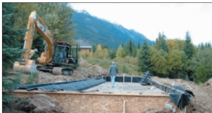
A sand filter nears final construction as the Infiltrator chambers are placed on the filter material. The chambers allow a better effluent dispersal and gas exchange.
