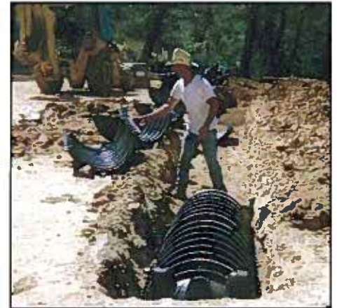
The septic system at Packers Bay Marina includes a drainfield with 624 feet of Infiltrator Quick4 Equalizer36 chambers. The chambers offered greater storage capacity for peak flows such as are common on summer weekends.
