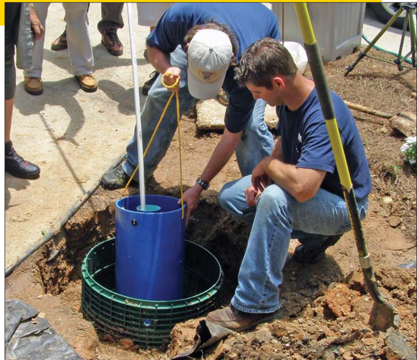
Brian Parker guides the Aquaworx Remediator into the septic tank. It must sit firmly on the bottom and below the riser for easy access. Matt Vinson looks on. (Photos courtesy of Infiltrator Systems Inc.)
