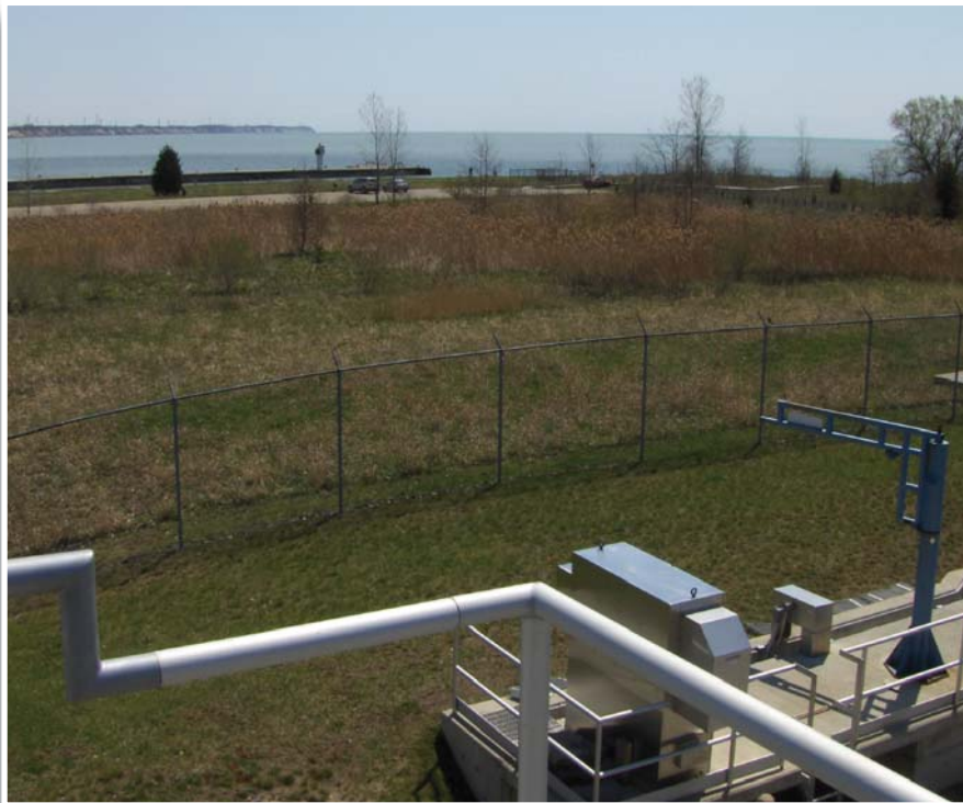
The Port Burwell Sewage Treatment Plant sits on the shore of Big Otter Creek near Lake Erie in Ontario. The system has more than met the original capacity projections and environmental requirements.
